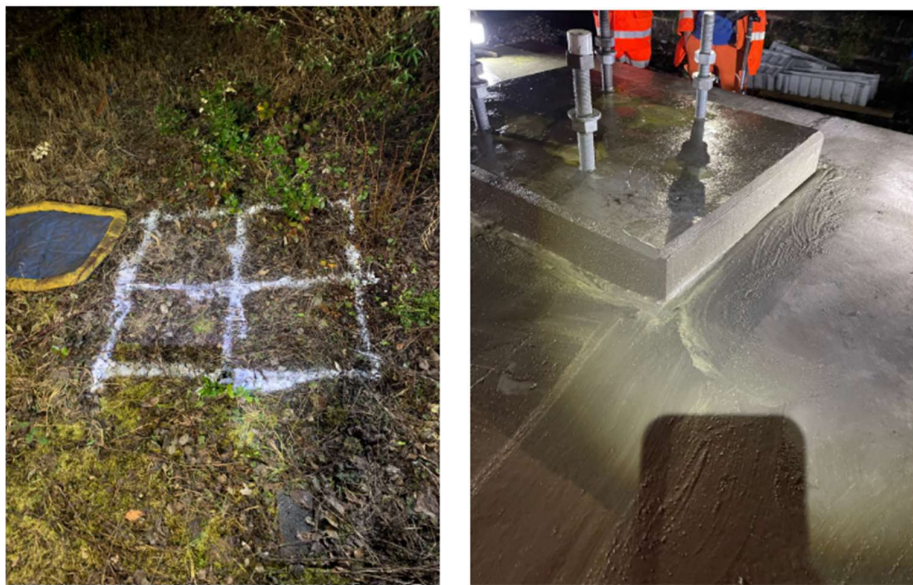
Figure 7-2: Installation of foundations and masts/support structures in preparation for the electrification works
